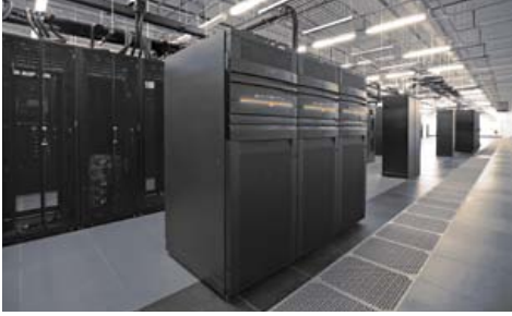
Power Loft uses a two-story design with the raised floor on the second story and the mechanical and air-handling equipment on the ground floor to maximize server rack space and improve cooling efficiency.
